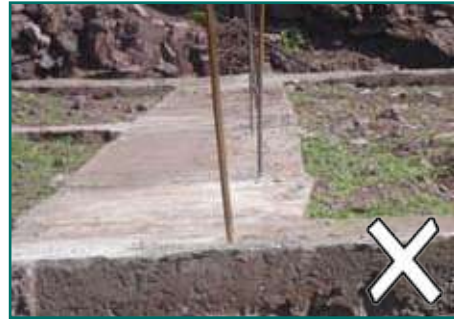
Wrong placement of vertical bars
