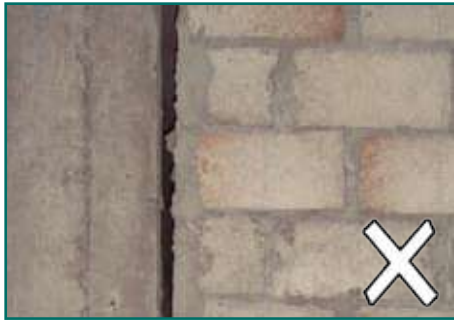
RCC columns cast first No connection to walls
