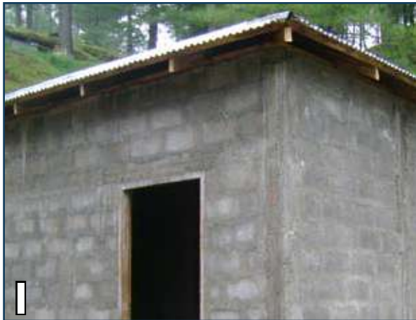
1 Continuous lintel and roof beam is missing.
