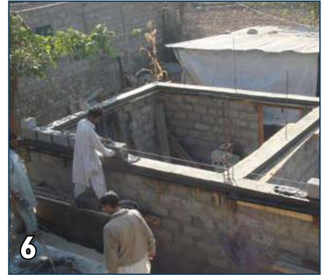
6 After initial 3 days of curing, construction above lintel band can be started. Repeat the same procedure for roof band.
