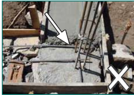
No connection at corners
