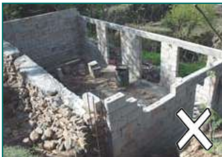
> 50% openings in a wall. Openings too large
