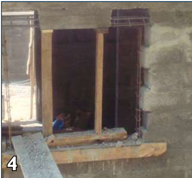
4 Prop the lintel band/beam and chisel 12" concrete of beam/ band for embedment of reinforcement.
