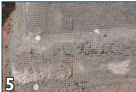
5 Fix wire mesh on concrete (beams and bands) with steel nails using bottle caps or #10 screws with 1" dia washers.
