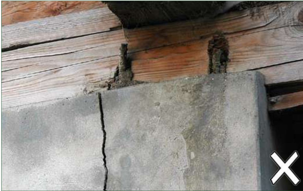
RCC column fixed to timber beam. This is not permitted.
