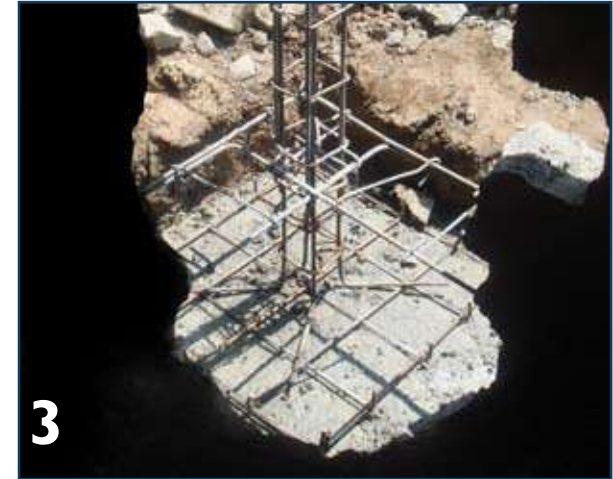
3 Dismantle plinth band/beam without damaging the reinforcement. Place reinforcement mesh and vertical column bars with proper feet.
