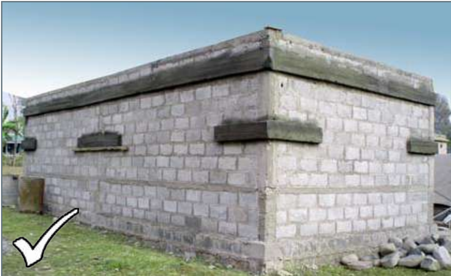
Method- 3: An external reinforced concrete band on both sides of the wall connected together by cross ties. For further details see Compliance Catalogue Appendix- A (External Band Flyer)
