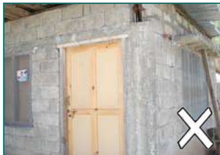
Openings too close to corner/ other openings
