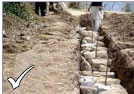
For timber frame/ dhajji construction the bolts should be fixed in foundation below natural ground level.
