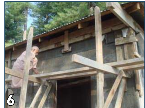
6 Place shuttering and pour 1:2:4 concrete in roof beam and cure for 10 days.
