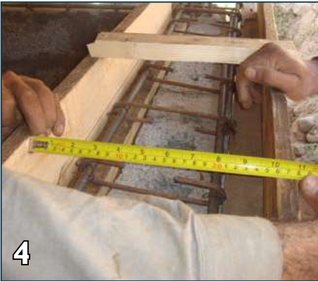
4 Fix shuttering on vertical faces and ensure the internal distance between vertical planks is 10".
