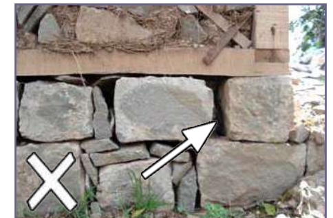
Plinth should not have gaps.
