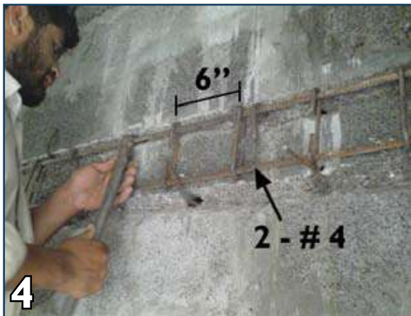
4 Place reinforcement at both faces and fix them firmly with 1/8" dia connectors.
