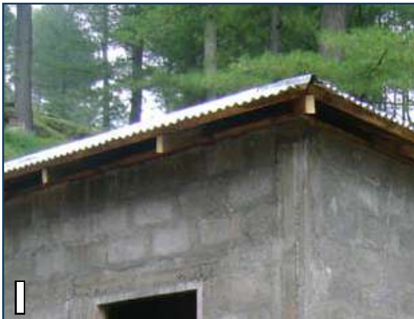
1 Continuous roof beam is missing.
