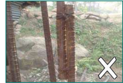
Insufficient overlaps for vertical reinforcement
