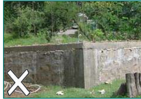
Plinth too high / unequal
