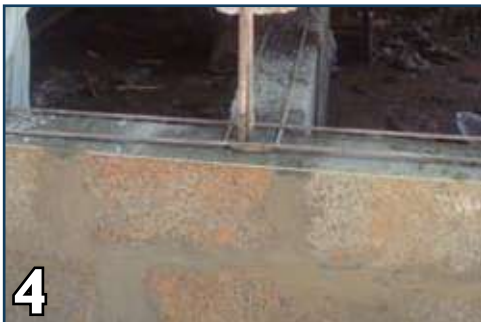
4 Lay masonry with 24" long stitches with 2- #3 bars after every third course (or max. 24").
