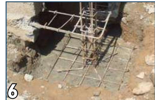
6 Extend column reinforcement with proper lap and proper foot to reinforcement pad in foundation
