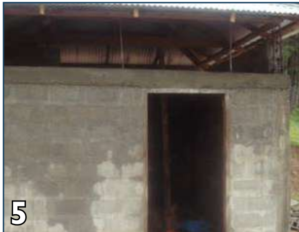
5 Pour 1:2:4 (cement:sand:aggregate) concrete for new lintel band and cure for at least 7 days.
