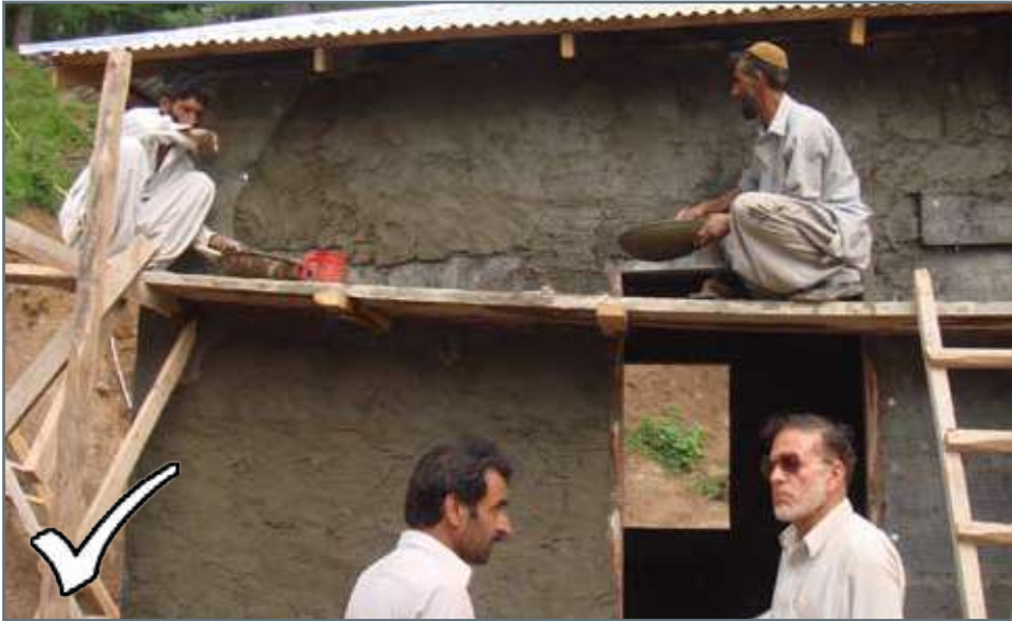
Method- 1: Plaster with wire mesh on both sides of the wall. For further details see Compliance Catalogue Section D (Remedial Measure)
