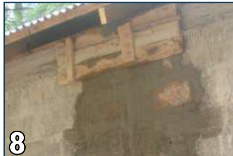
8 Place shuttering and pour concrete to replace dismantled portion of roof band.
