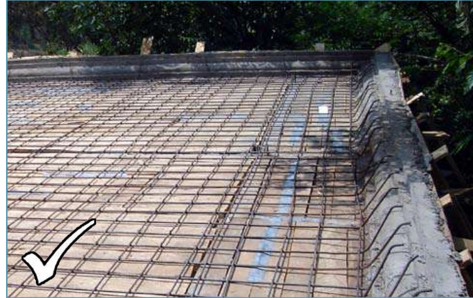
Reinforced concrete parapets up to 3ft height adequately integrated with RCC slab may be acceptable.
