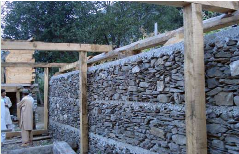
Timber posts inside and separate to the wall. RCC bands between well laid dry stone masonry.
