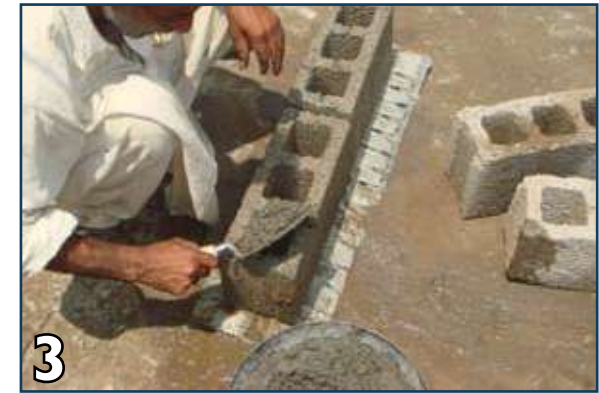
3 Pour 1:3:6 concrete mix in layers in the cavities (fill one cavity at a time).
