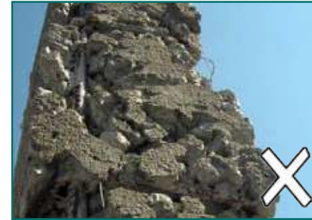
Exposed reinforcement bars
