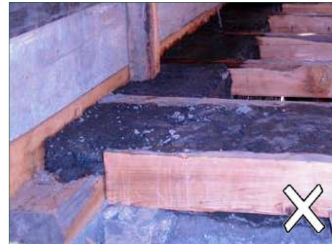
Heavy insulation in the roof is dangerous.
