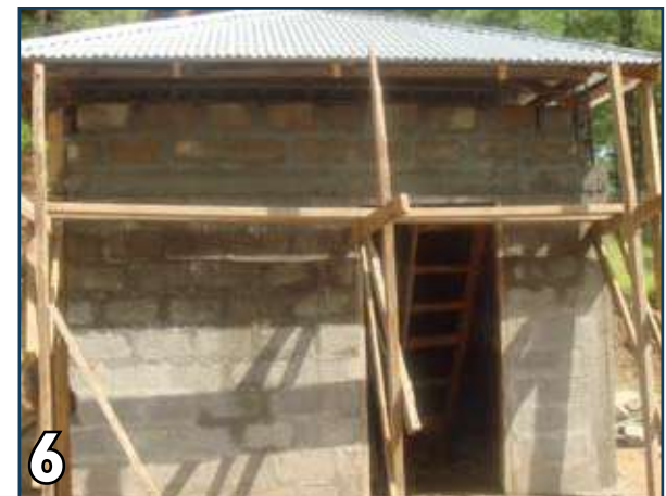
6 Lay masonry over newly casted lintel beam, in case of confined masonry provide tothing at the corners and provide roof beam at the top.
