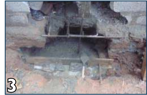
3 Place #4 or #5 bars over P.C.C. passing through bands. Place shuttering and pour concrete.
