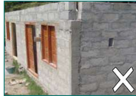
Horizontal bands missing
