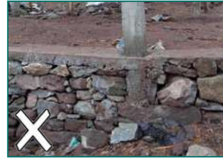
No anchorage to columns
