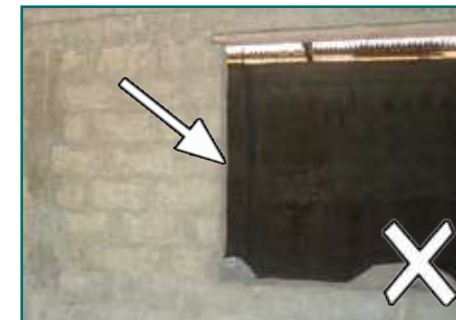
Openings without framing reinforcement
