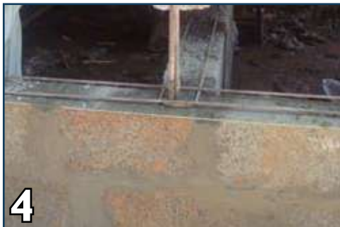
4 Lay masonry with 24" long stitches with two #3 bars after every third course.
