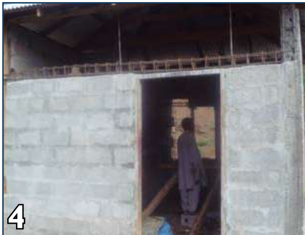
4 Place 4-#4 continuous reinforcement with #3 @ 6" spacing stirrups for lintel beam with adequate connection with vertical reinforcement bars and confining columns.
