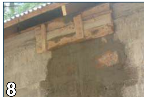
8 Place shuttering and pour concrete to replace dismantled portion of roof beam/band.
