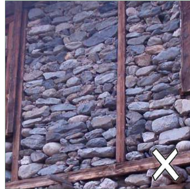
Stonework with no bracing.
