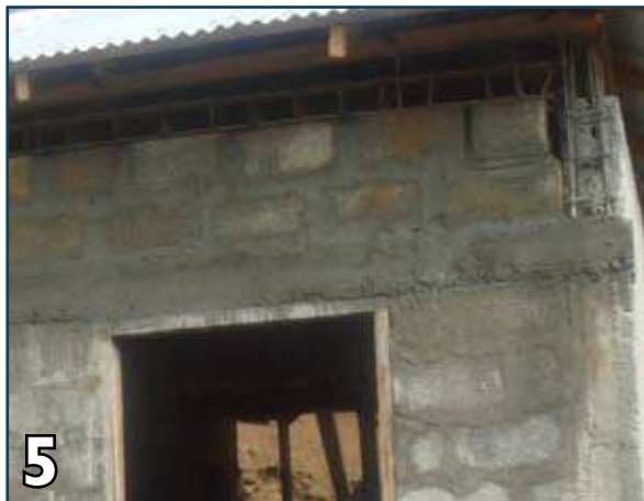
5 Place 4 #4 continuous bars with #3 @ 6" spacing stirrups for roof beam with adequate connection to vertical reinforcement bars and confining columns.
