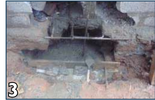
3 Place #4 or #5 vertical bars over P.C.C. Passing through all bands. Place shuttering and pour concrete.
