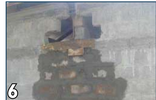
6 Place shuttering and pour concrete in existing chiselled and new lintel beam/band.
