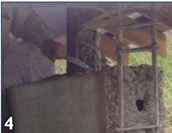
4 In case of confined masonry chisel the upper part of the columns to have proper connection between roof beam reinforcement and columns.
