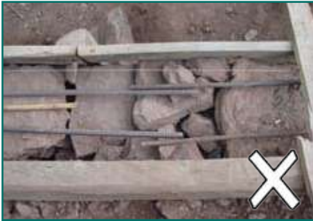
Insufficient overlap of reinforcement bars
