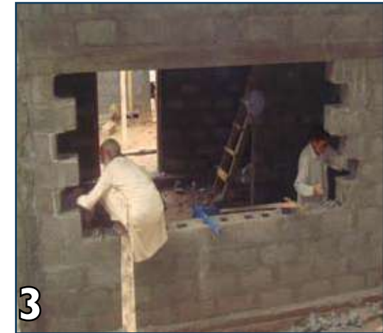
Provide tootthing on either/both ends to reduce the opening or increase the distance from the corner.
