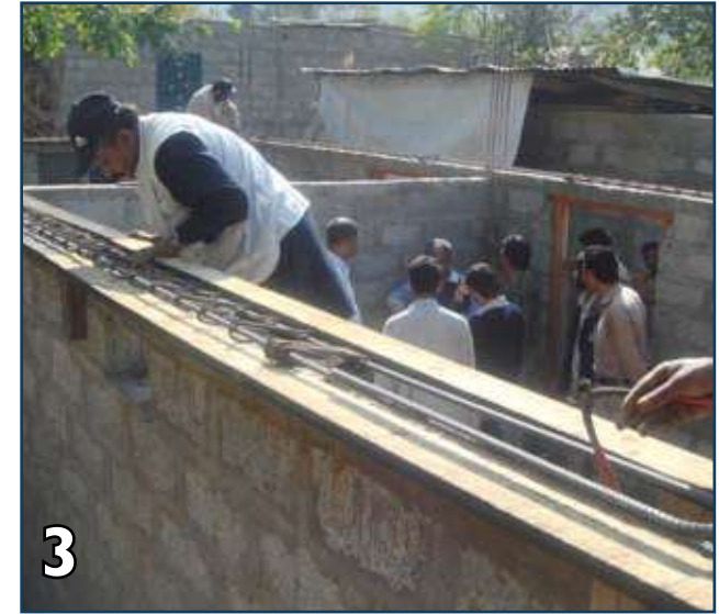
3 Fix the bottom planks of shuttering on both sides of the walls and fix reinforcement properly.
