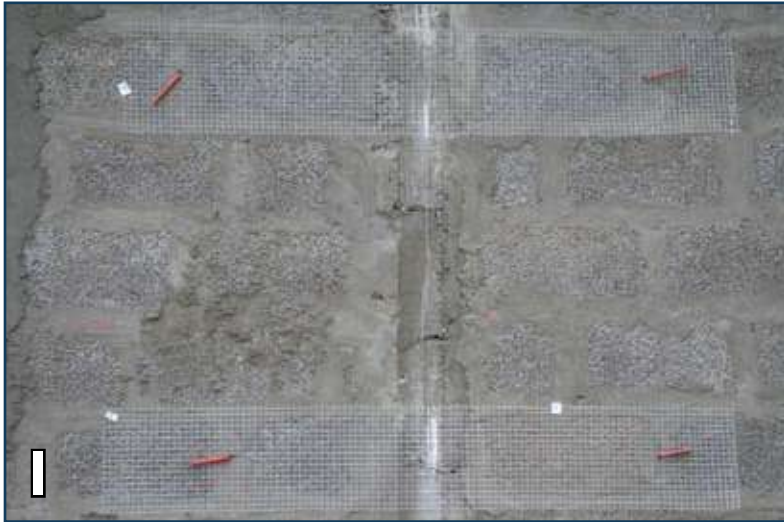
1 Drill holes and fix mesh after every three courses on both faces of the wall with 1/8" dia connectors.
