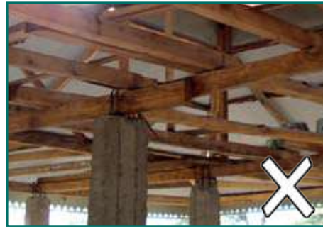
Free standing columns No connection to roof beam
