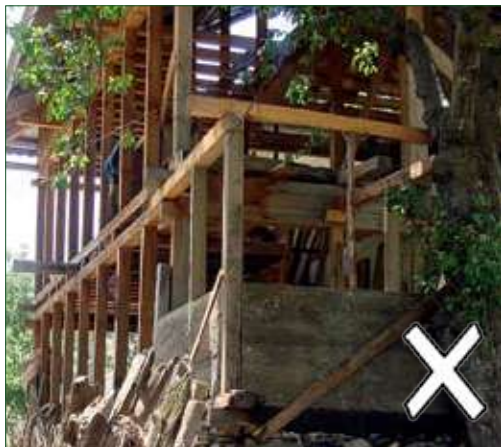
Even small areas of in situ may weaken the frame.
