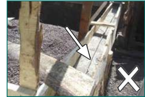
Insufficient reinforcement in bands
